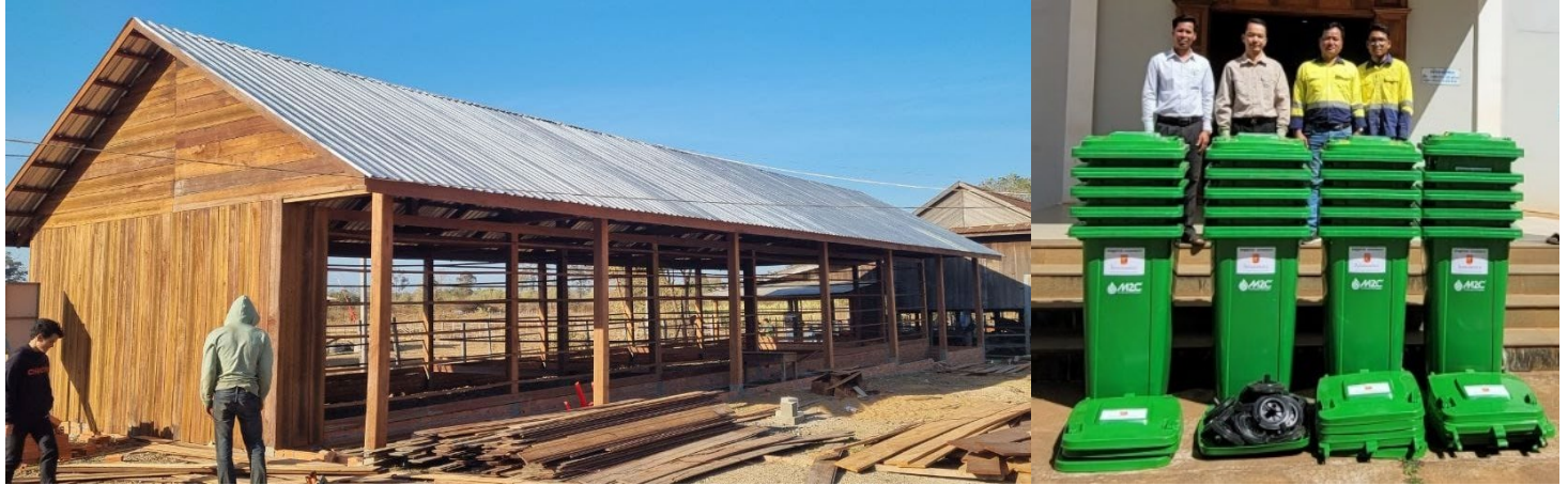
Figure 29 | Initiatives supported this Quarter include a new roof for a school and donated waste receptacles
