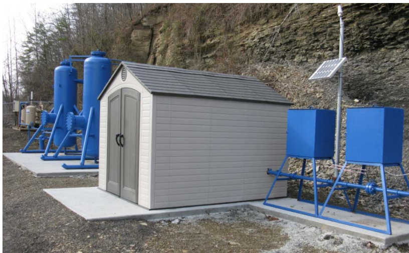
Beetree Gas Compression and Sales Gas Treatment Facilities
