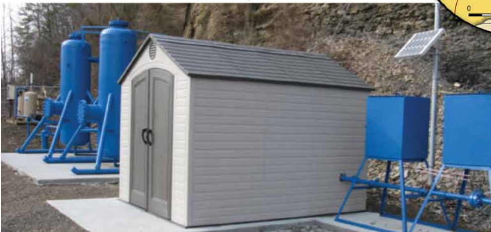
Beetree Gas Compression and Sales Gas Treatment Facilities
