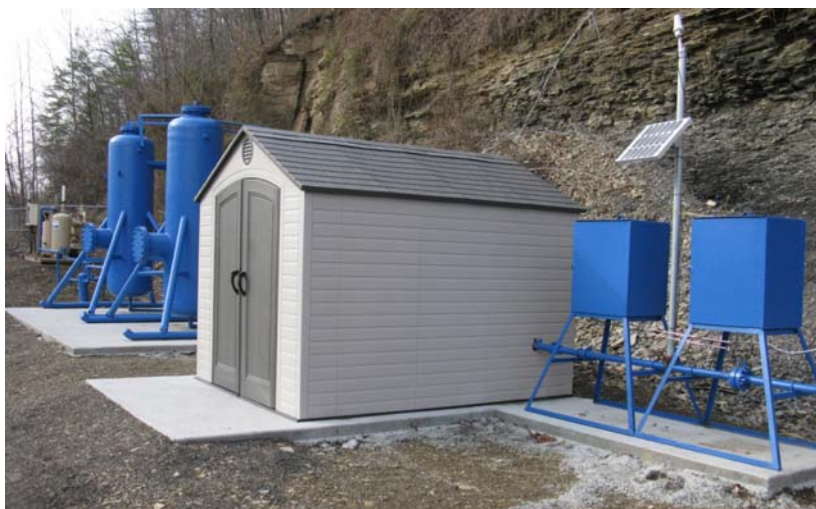
Beetree Gas Compression and Sales Gas Treatment Facilities
