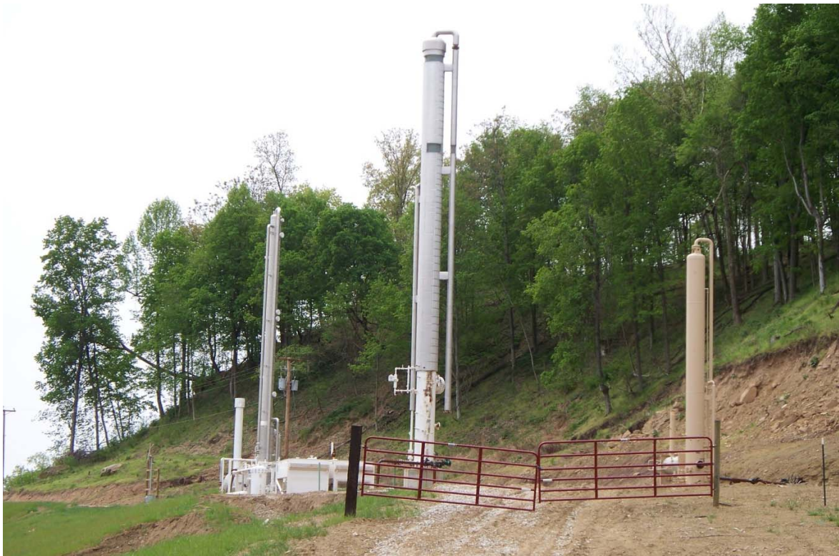
P&J Resources' Amine Plant in Wayne County West Virginia.
