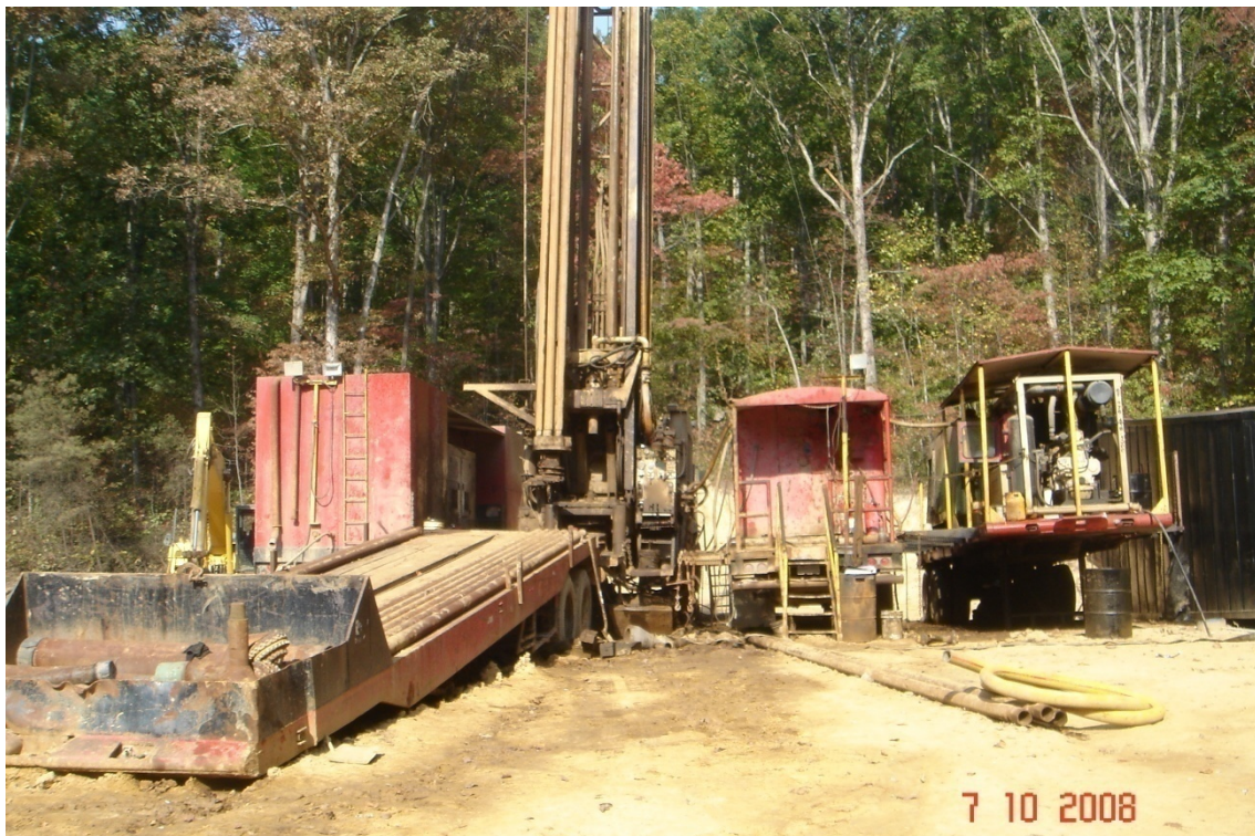
Drilling rig on location at Chiarenzelli 1 well site, Wayne County West Virginia.
